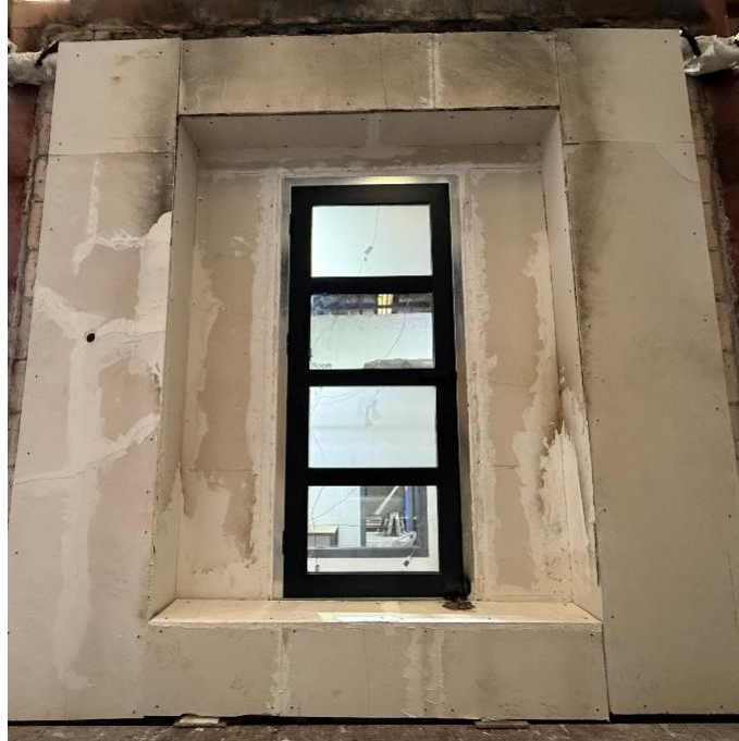
Fig. 3 Fire exposed side after 60 minutes
